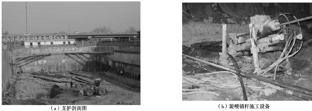
图 2 地铁五号线雍和宫车站旋喷锚杆 Fig. 2 Jet-grouting self-boring anchors in subway Line 5
