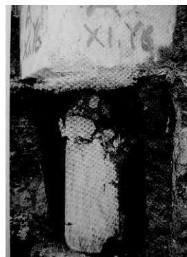
(a) 阪神地震中桩头破坏
